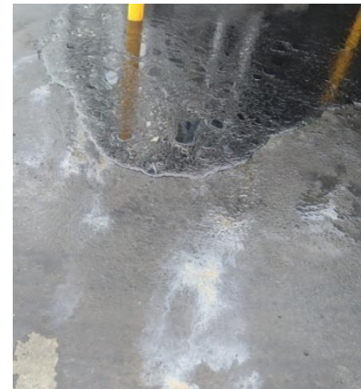
Bitumen Spill – Oily run off
