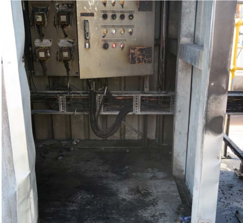
Image 3.11 Damage inside switchboard shed.
