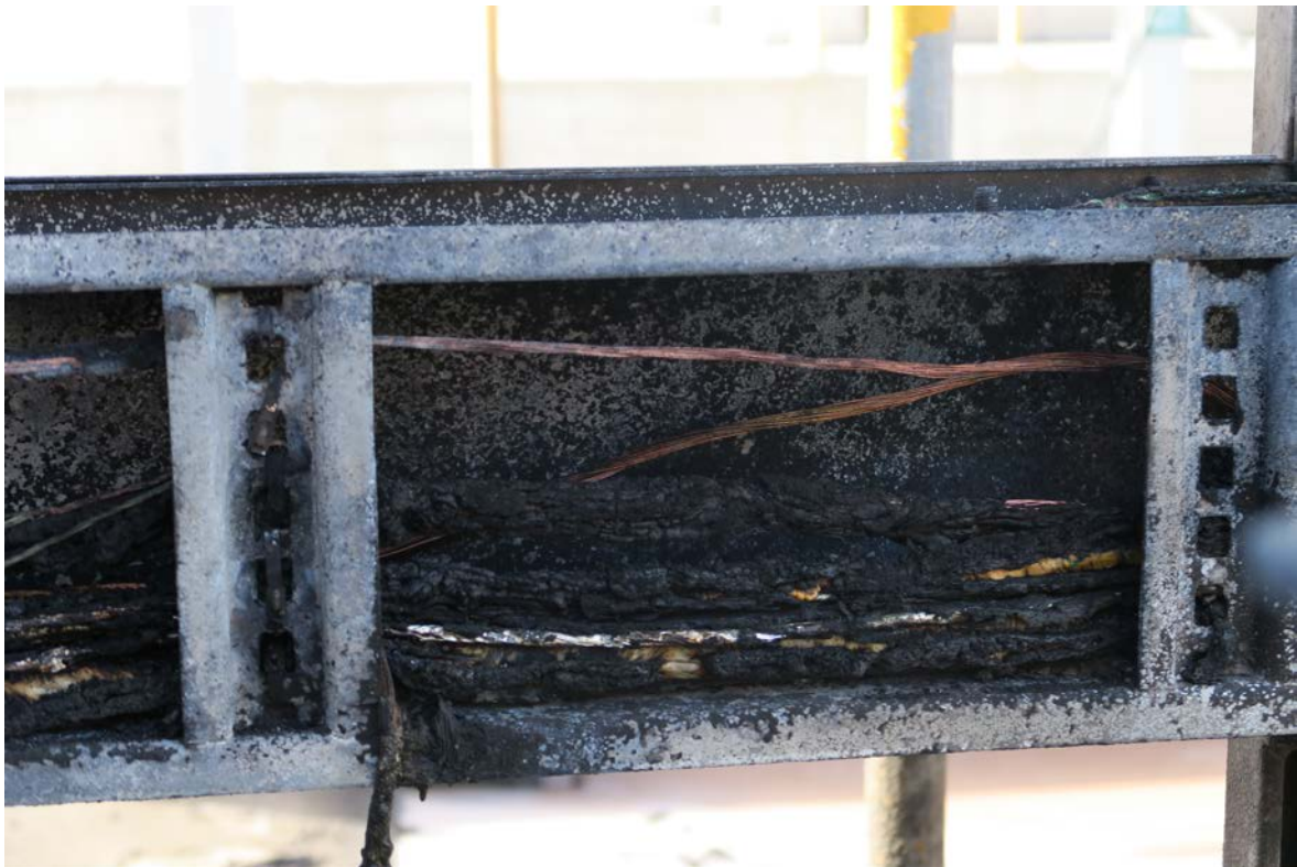
Image 3.12 - Damage to wiring leading into switchboard shed.
