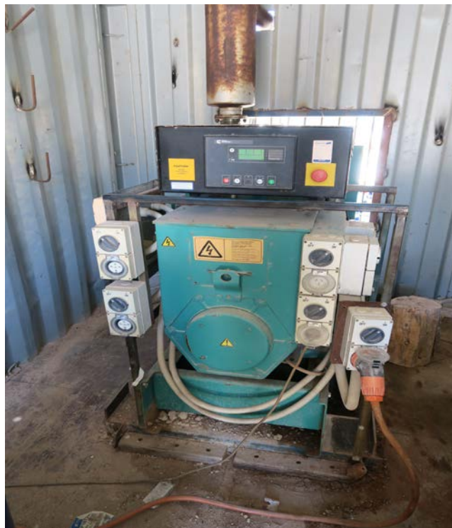
Figure 12: The generator that powers the electric motor to the hydraulic system and underground lights.
