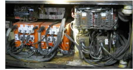
Open control panel exposing electrical connectors.
