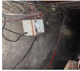
Work performed inside an energized enclosure.
