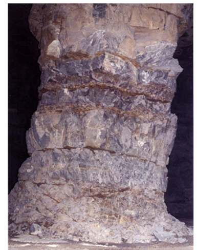
Be Alert for Spalling and Hourglassing
