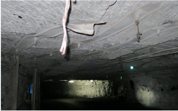
Figure 12: Damaged W straps the vicinity of the incident.
