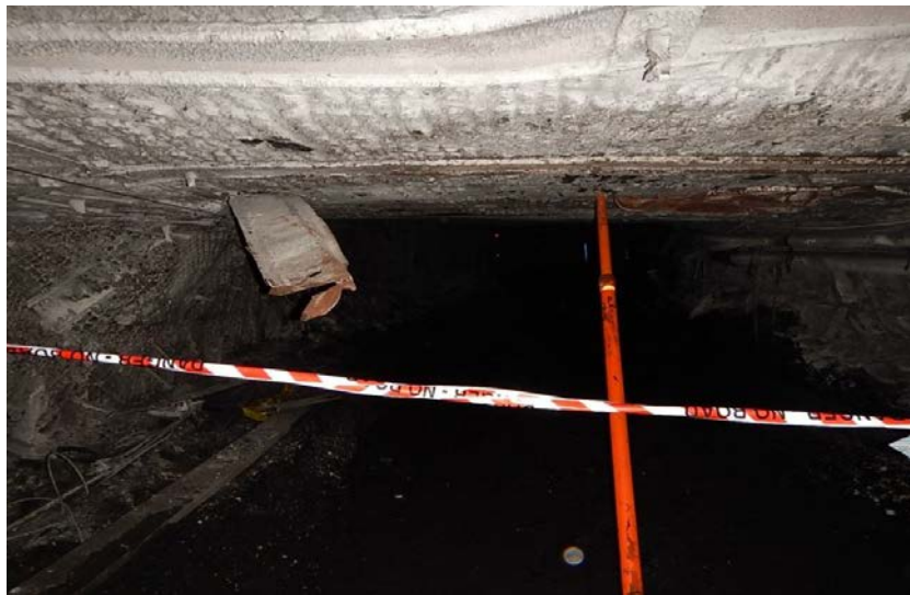
Figure 13: The incident scene looking inbye at the damaged W strap hanging from the roof.
