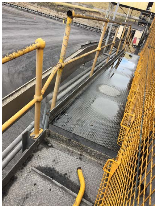
Figure 33: Handrail corroded and fallen off.
