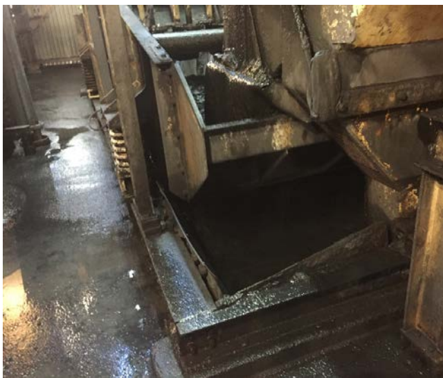
Figure 31 and 32: No protection against falling into screen underpans.
