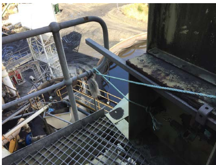
Figure 34: Rope and unistrut are ineffective to prevent falling.
