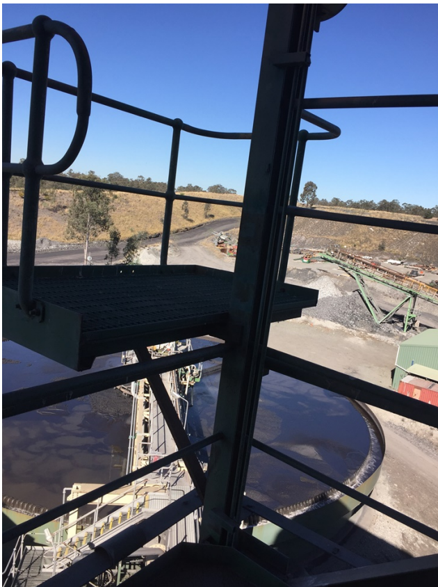
Figure 25: Access platform added without ladder.
