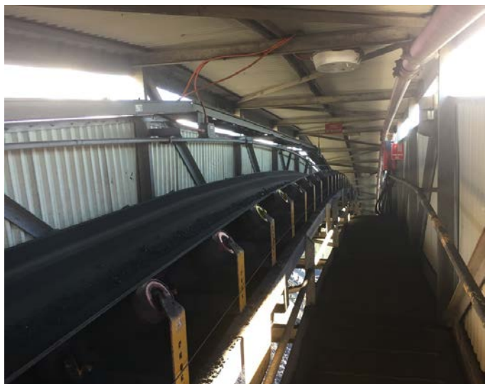
Figures 59 and 60: Guarding of conveyor brow rollers.
