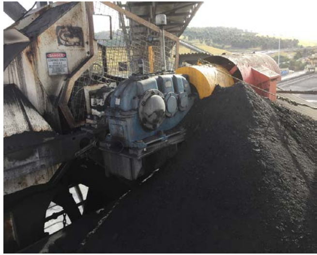
Figure 50: Fine dust build-up on pulley bearing guard.
