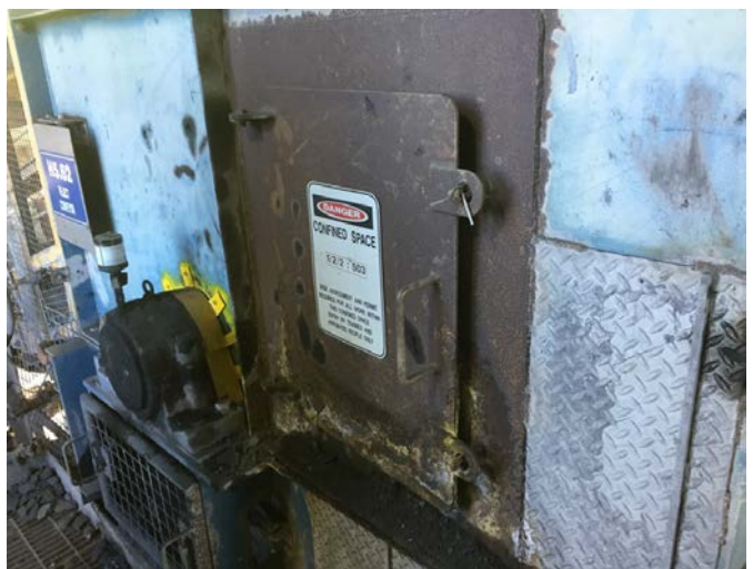
Figure 14: Access hatch beside pulley nip point not secured.
