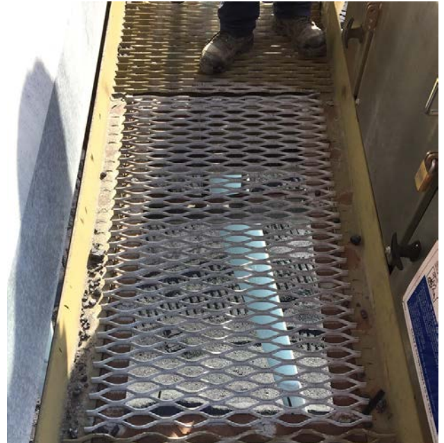
Figure 24: Section removed from walkway not secured.
