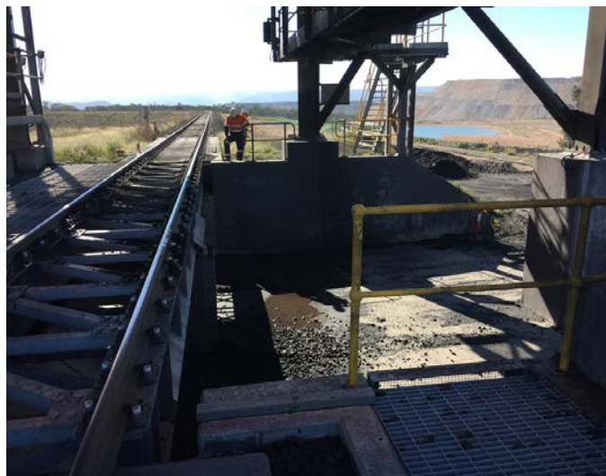
Figure 28: Handrail does not fully protect against falling
