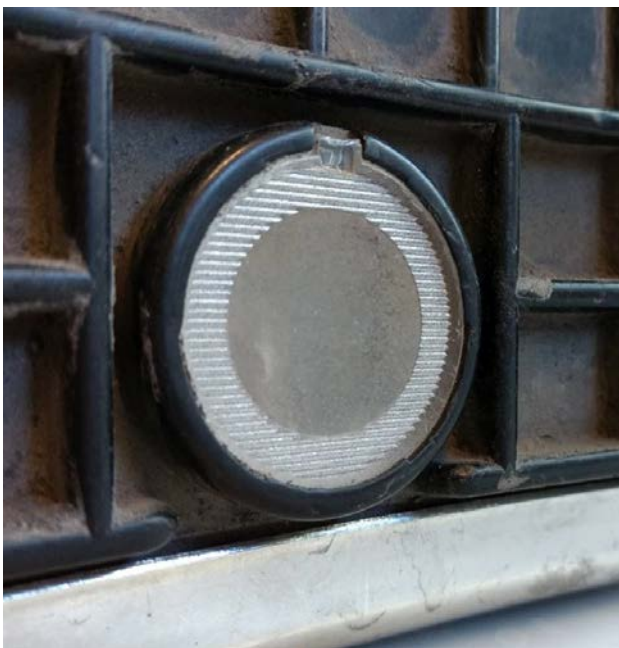
Photo 1: Dirt obscuring the moisture indicator.
