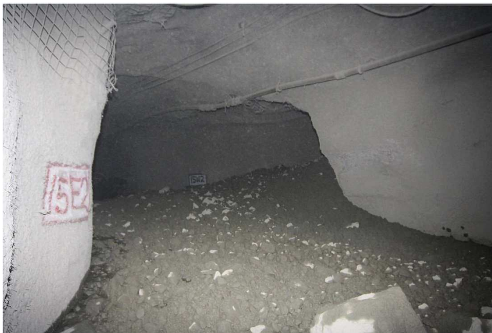
Figure 18 An uncontrolled inflow of wet material at a draw point in extraction drive 15 in August 2015.
