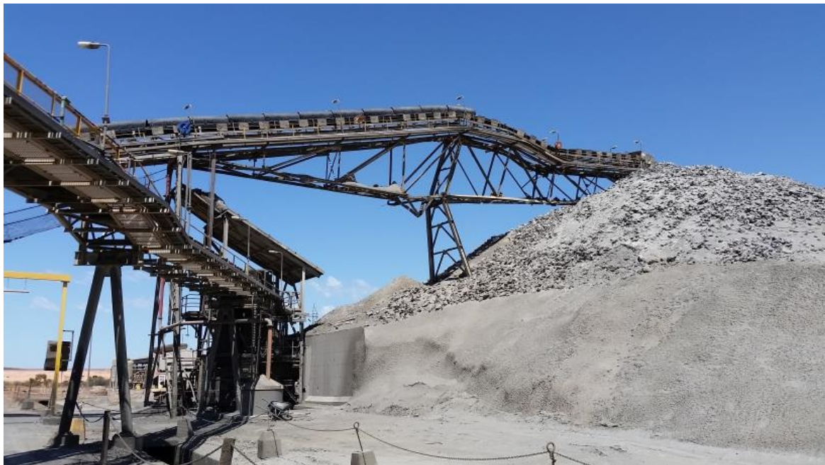
Collapsed stacker resting on stockpile and showing product build-up on bottom chord.
