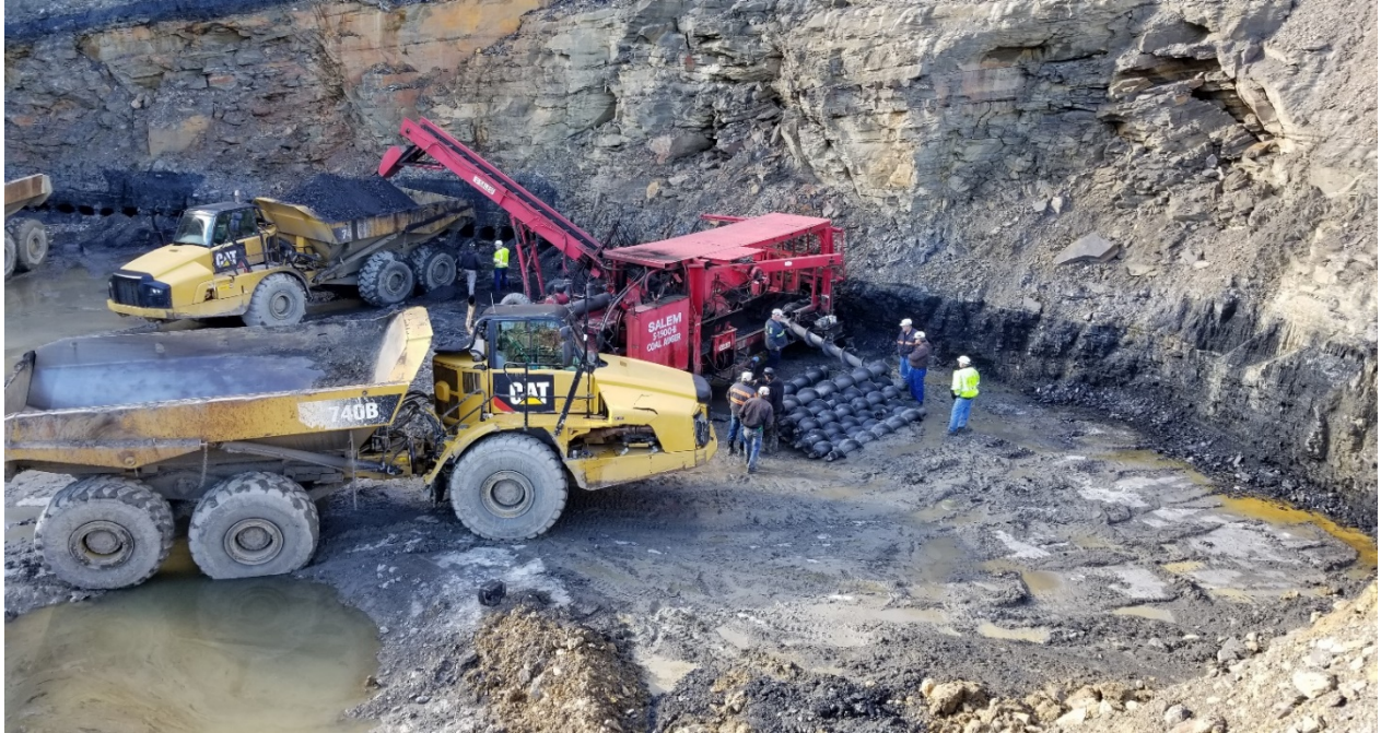
Photograph of Accident Scene
