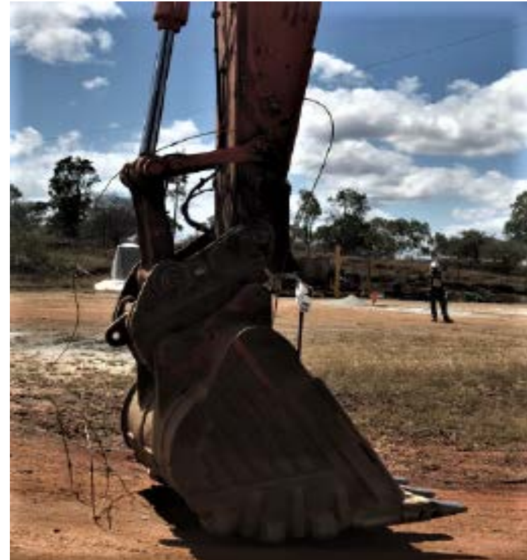
Conductor entangled around excavator boom
