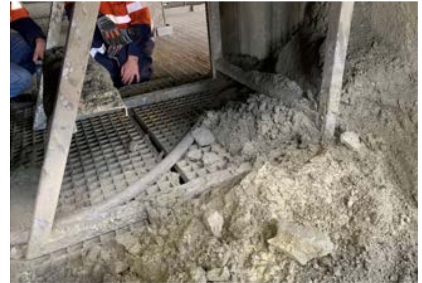
Inside the chamber after the incident
