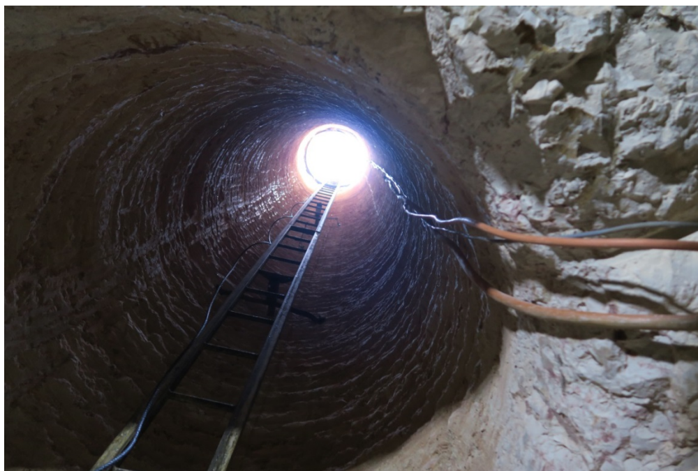
Photograph 3: The shaft, guide rail system, steel cable and electrical cable (taken from the base of the shaft).
