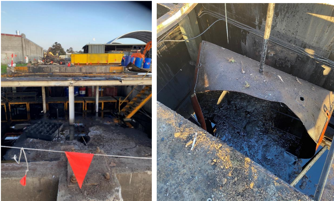
The pit where the explosion occurred and the tank that ruptured.
