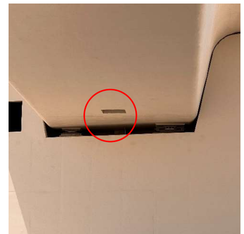
Worker fell through opening here
