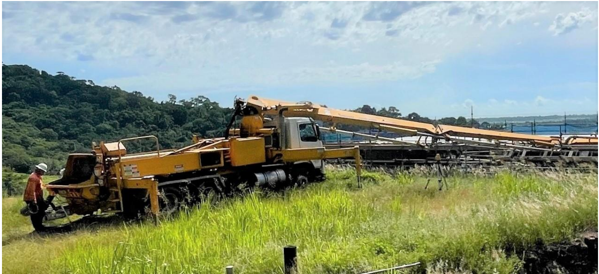
Photograph 1: Mobile concrete placing boom with a collapsed boom.
