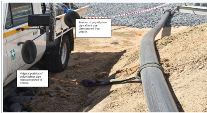
Example of a sudden release of stored energy
