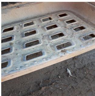
Footplate in poor condition
