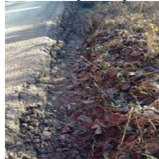
Rut to side of road
